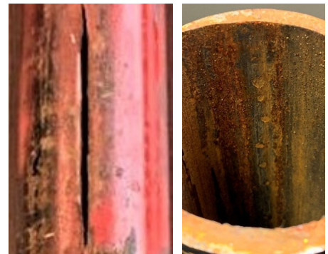
Tubing Failure and Erosion
