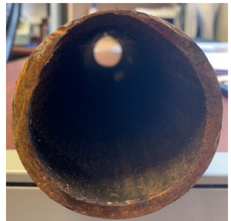
Major Wall Loss
