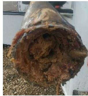
Wax Build-Up in Regular Tubing String After 10 Days
